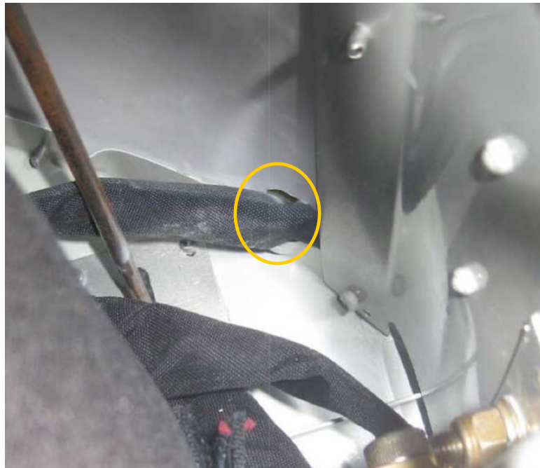
Figure 6: picture taken from an installation inside showing the hole in the egress panel
